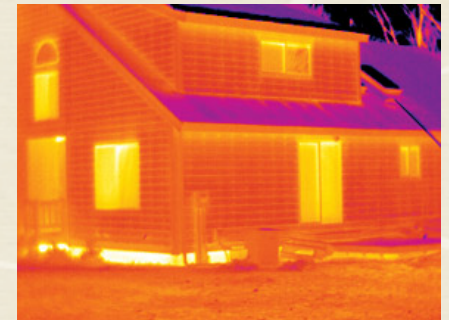
Yellow and orange areas of damaged deteriorated roof are barely visible in daylight
